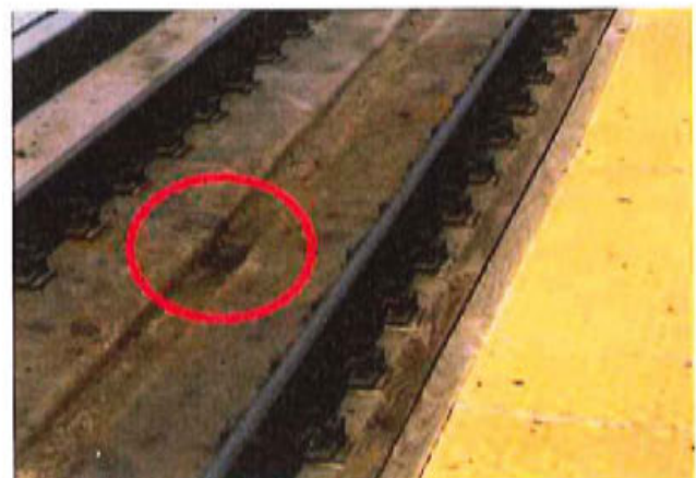
Figure 7. Water Infiltration between the Rails
