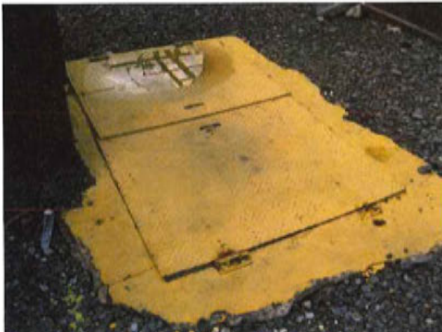
Figure 37. Control Pit Flooded During Hurricane Sandy
