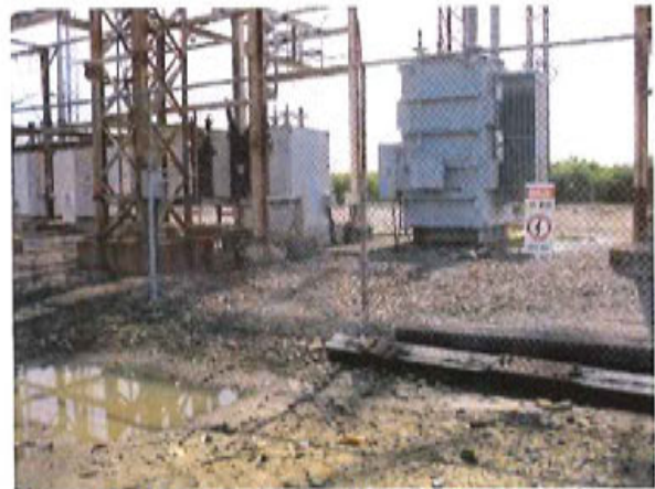
Figure 32. Water Ponding at Bellevue Substation
