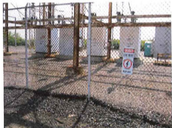
Figure 33. Substation Equipment on Elevated Concrete Footings
