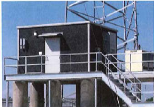
Photo Credit: Modular Connections; modularconnections.com/communication-shelters/
