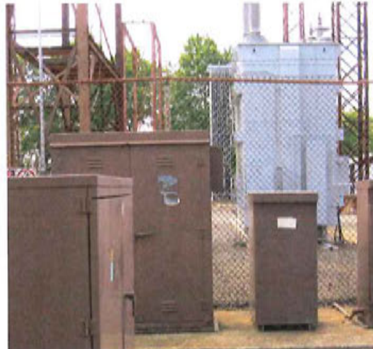
Figure 36. West Yard - Substation Equipment
