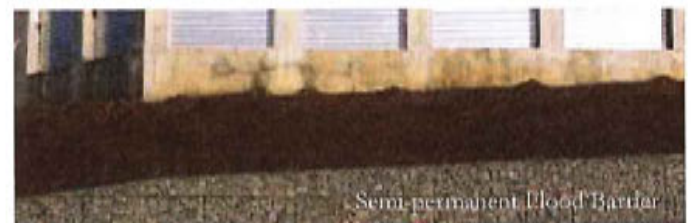
Permanent Flood Barrier
